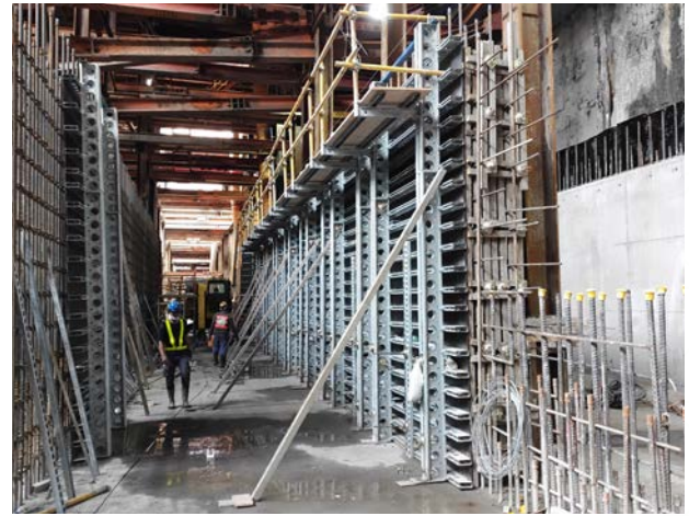
Taipei Metro WanDa Line 1st Phase CQ872 Compartment Wall 4.5M High Double-Sided Wall Formwork
