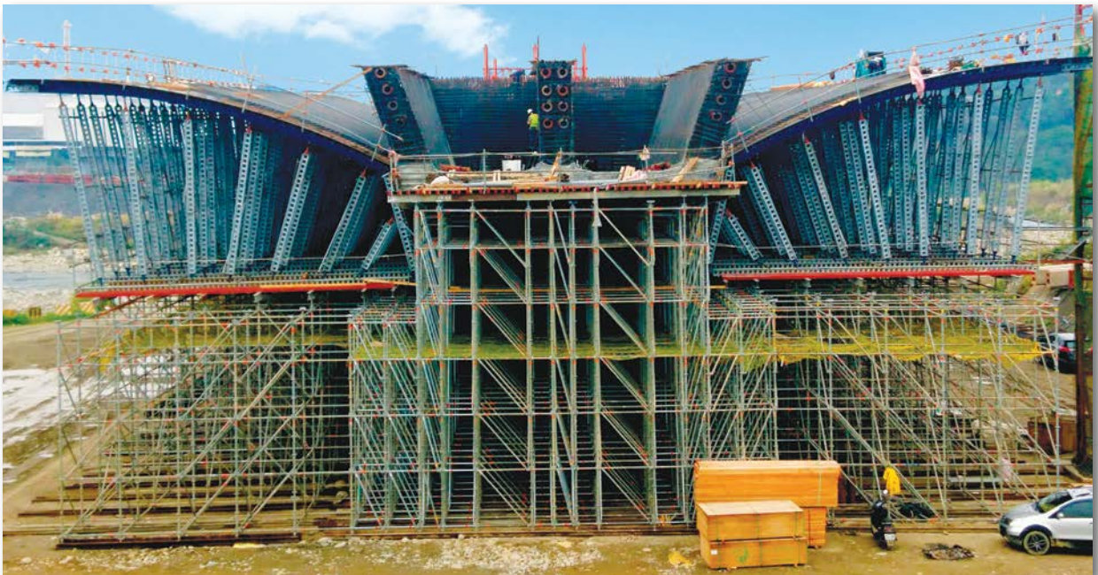
Top Beam connected with Base Beam as Second Bearer on an external formwork of superstructure of bridge formwork project
