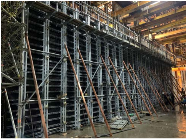
Taipei Metro WanDa Line 1st Phase CQ852 Compartment Wall 6M High Double-Sided Wall Formwork
