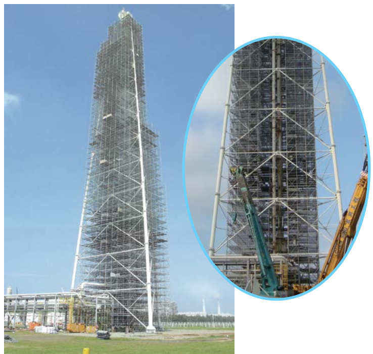
FPCC No.6 Naphtha Cracking Project (140m Height)
